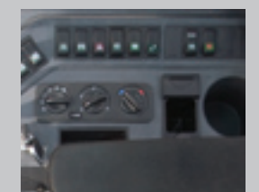
Instrument Switch Panel
